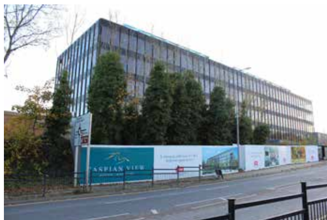
Mercury House - a 1980s office building, designed by Milton Keynes Development Corporation and currently being converted into apartments
